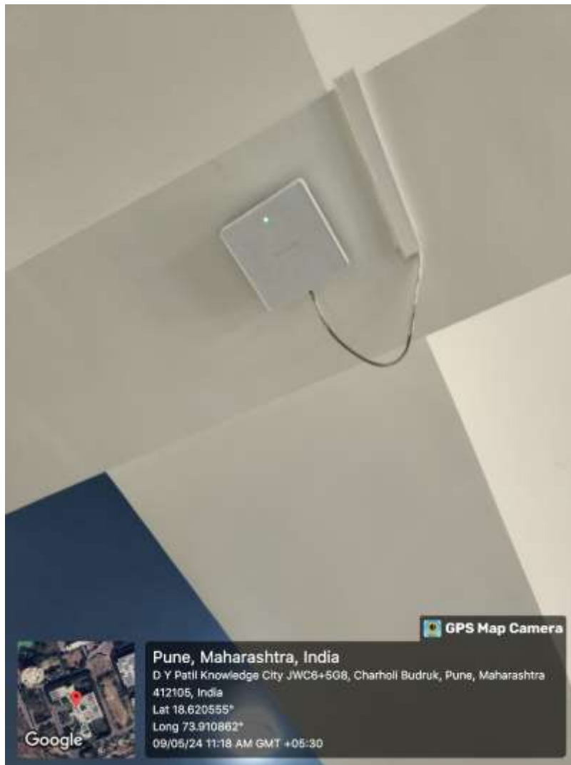
Wi-Fi Router in the Prosthodontics clinical area located on the First floor of the Hospital Building
